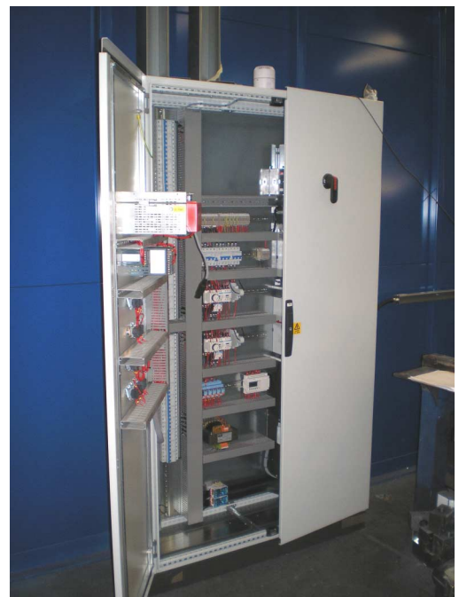
The control system
